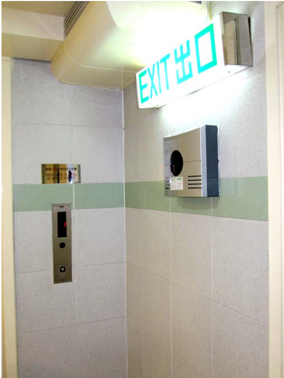
Innoclean – Purezone R601 at Lift Lobby:
