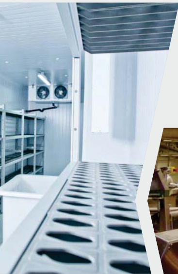
Cold storage cells Blast chilling cells
